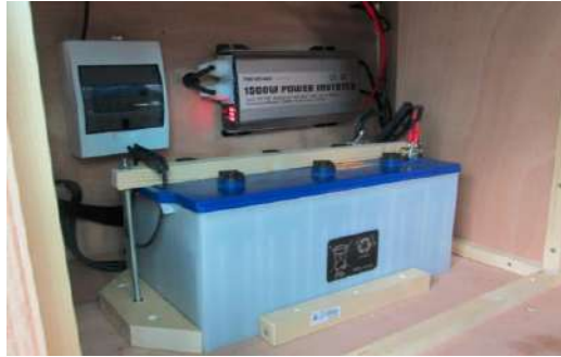
Figure 6-6 – Power supply for the set-up (battery and inverter)
