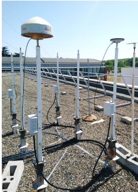
Figure 4 – Photos of the choke-ring antenna on the roof of an ENAC building
